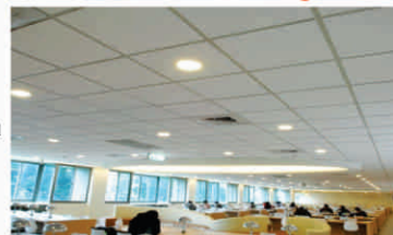
T-Grid False Ceiling
